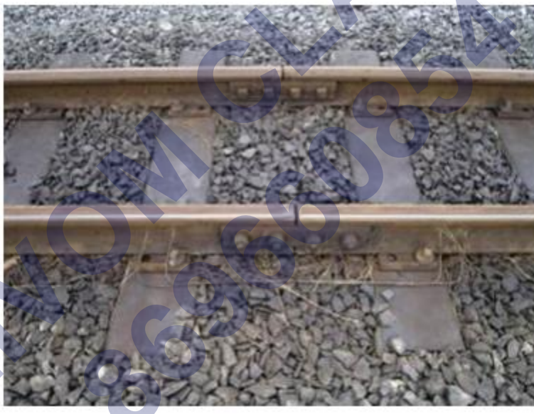
Small gaps between rails on the railway track.
