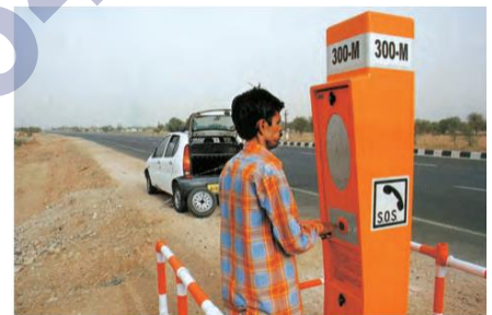
Emergency call box on NH-8
